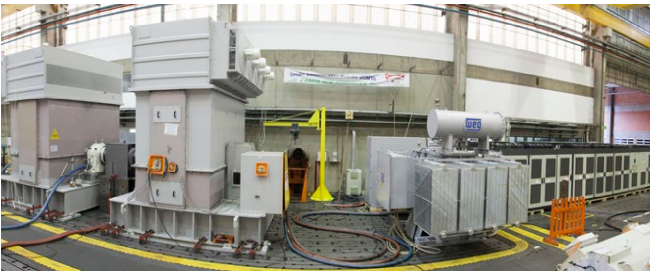
Combined test (MV Incoming Switchgear + Phase-shifting Transformer + MV VSD + MV Motor).
